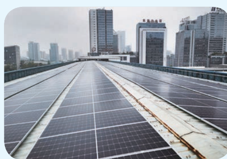
Photovoltaic facilities at Yao Pharma
