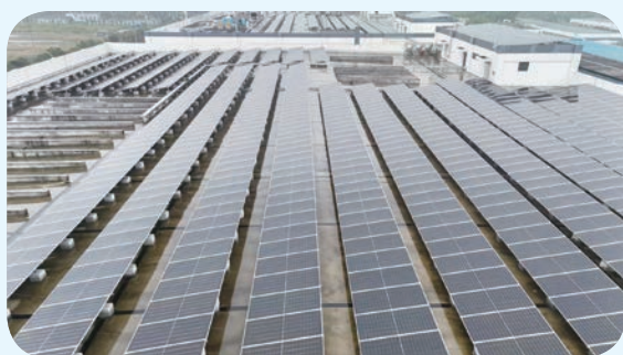
Photovoltaic facilities at Huaiyin Medical
